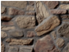
Chardonay Old Country Fieldstone (CSV-368105) Overgrouted mortar joints
