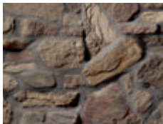
Chardonnoy Old Country Fieldstone (CSV-368105) Overgrouted mortar joints
